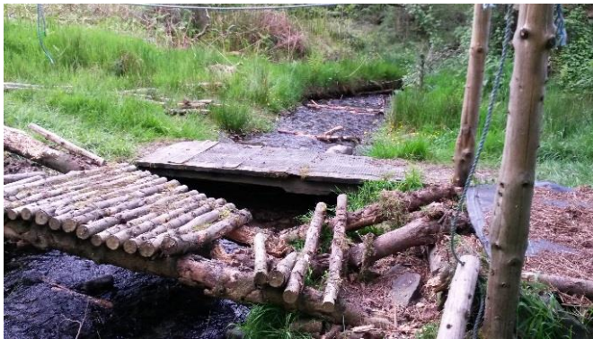
← Picture of left shows damaged bridge.
